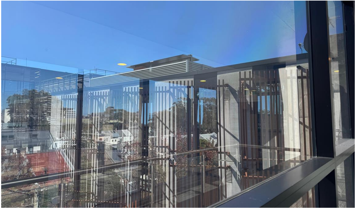
Figure 10: View of existing plant on roof
